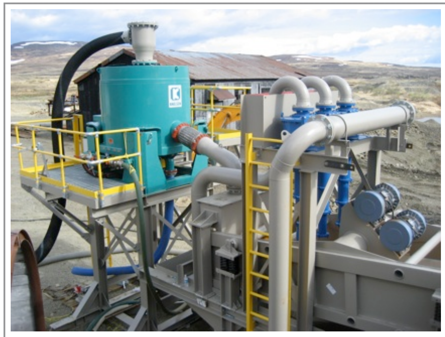
Phase 1 Knelson Concentrator & dewatering screen
